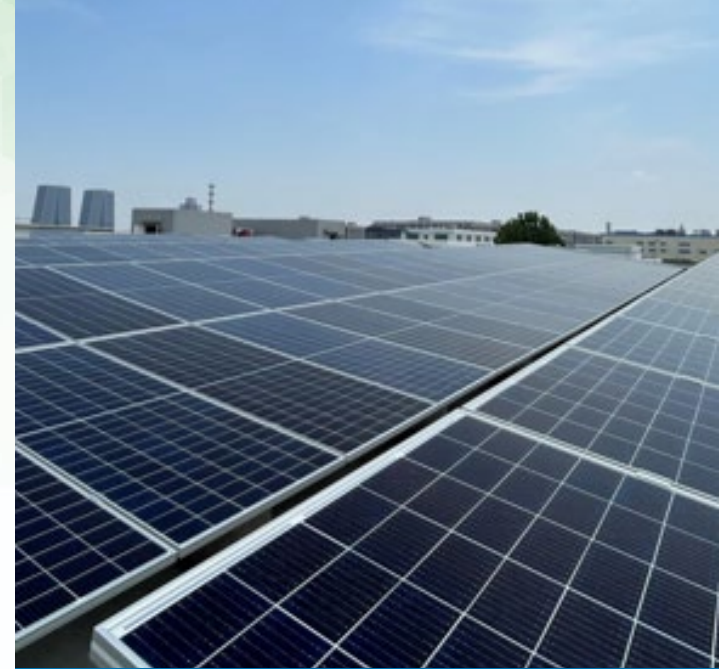
Solar panels installed on the MSA Suzhou China facility.
