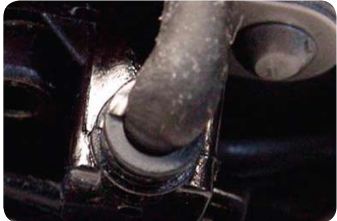
Value grade hub sensor suppliers claim their sensors will pass rigorous testing. Their sensors showed a direct path for water ingress, compromising sensor function.
