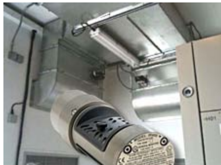
HVAC Gas Detection
