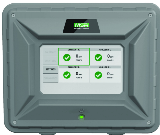
Fig. 13 Chillgard 5000 Remote Display
