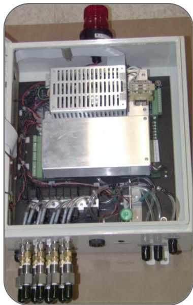
Interior, Chemgard Gas Monitor
