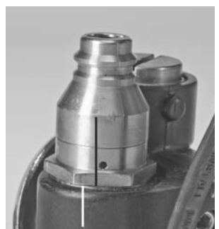
FIGURE 4 Loose at Manifold
