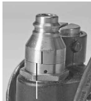
FIGURE 3 Loose at Coupling Joint
