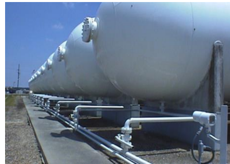
Figure 13: Leak point monitoring of a row of valves at a LPG storage area
