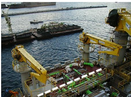
Figure 12: Leak point monitoring of offloading nozzles at a FPSO LPG offloading area
