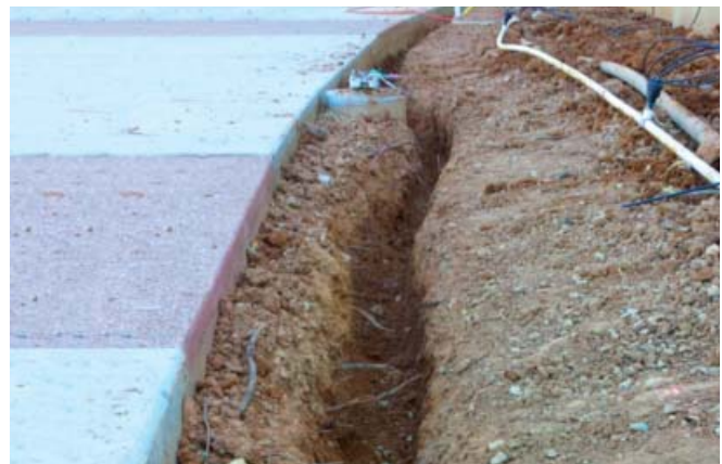
Excavating an area for sample line to monitor potential underground residual hazardous gases
